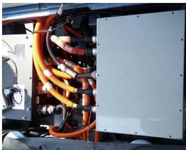
Figure. 7 Drive controller front installation
